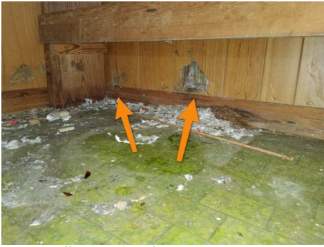
East wall varmint damage
