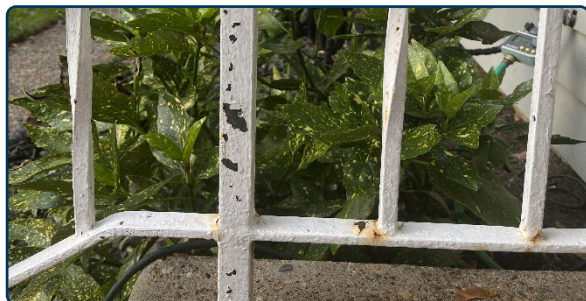
Figure 113: Metal railing in need of repainting to protect the railing.
