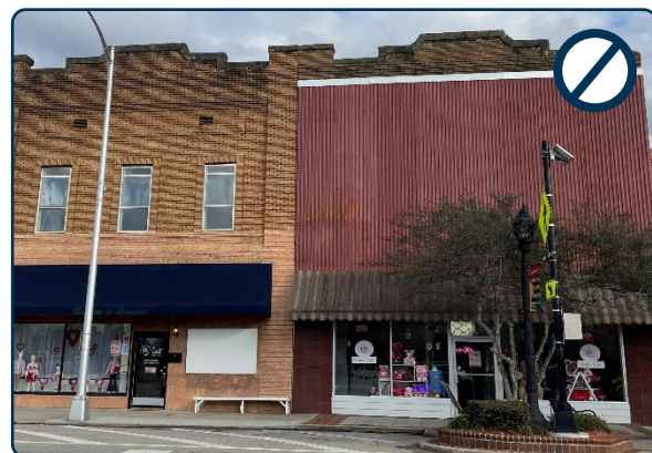
Figure 68: Inappropriate siding covering historic masonry on a commercial building.
