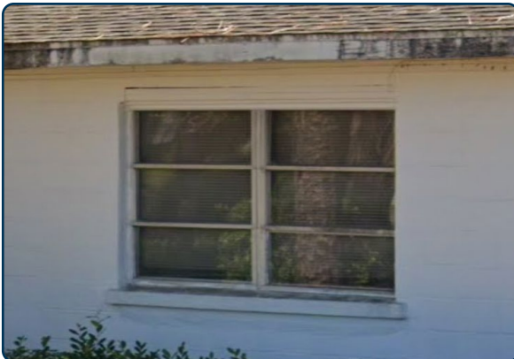
Figure 47: Historic residence that features wood windows and roof fascia that should be repainted and maintained.
