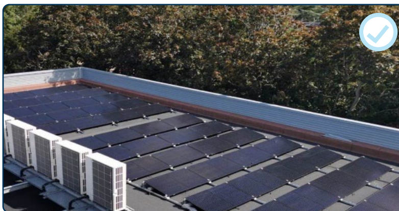
Figure 134: Solar panels installed on a flat roof obscured by parapets (Source: ESD Solar).
