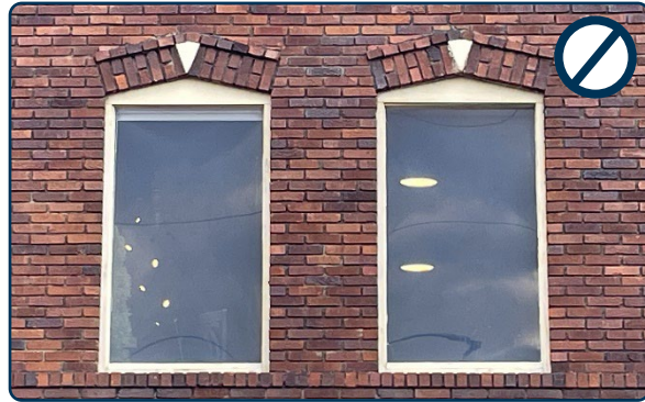
Figure 84: Inappropriate replacement window type that lacks appropriate muntins and meeting rails.
