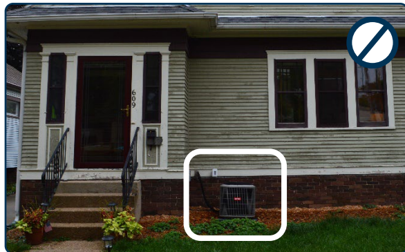
Figure 102: Inappropriate new air conditioner installed on the front façade of a residence that is not obscured behind screening or landscaping.
