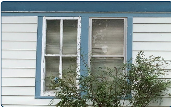
Figure 126: Inappropriate replacement window (right) that doesn't match the original.
