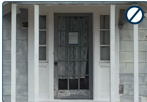
Figure 64: Example of a historic wood door needing to be re-painted.
