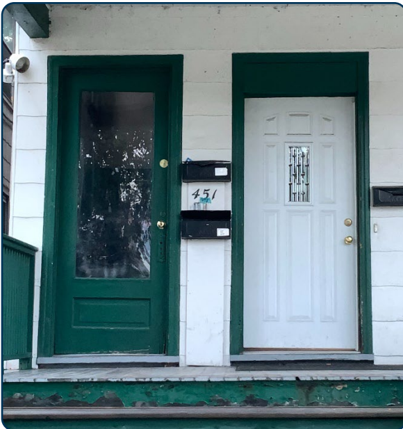
Figure 142: Inappropriate replacement door (right) that does not convey the architectural style of the residence.
