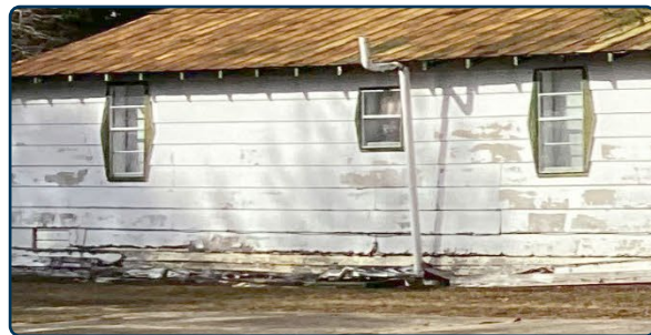
Figure 50: Historic residence that features wood siding visible under deteriorating asbestos siding.
