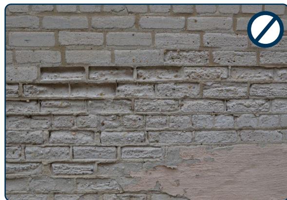
Figure 69: Inappropriate modern mortar replacement on a historic masonry building resulting in damaged bricks.
