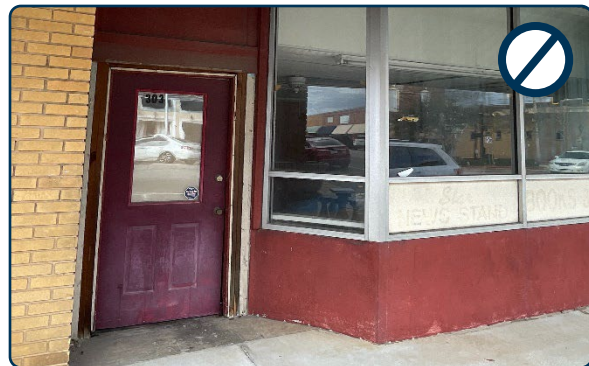
Figure 81: Inappropriate replacement storefront door that doesn't match the building's fenestration.
