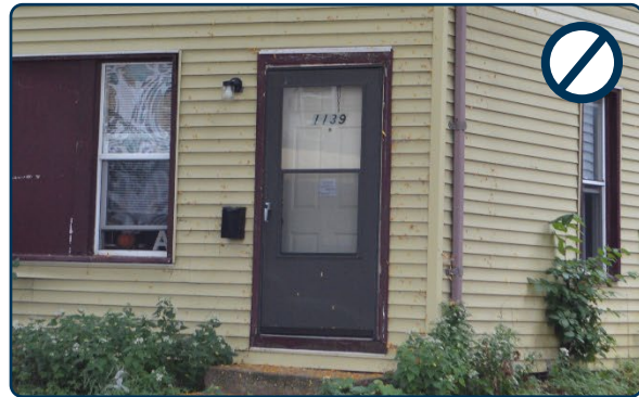
Figure 64: Inappropriate storm door that obscures the original door.
