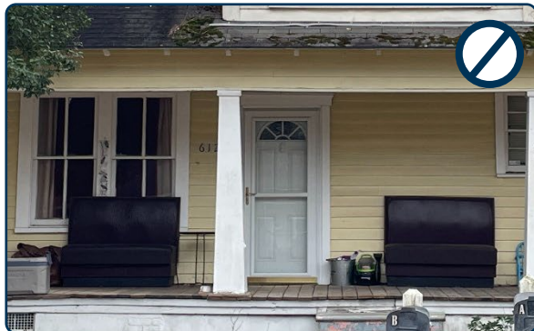
Figure 75: Inappropriate replacement of a historic door.
