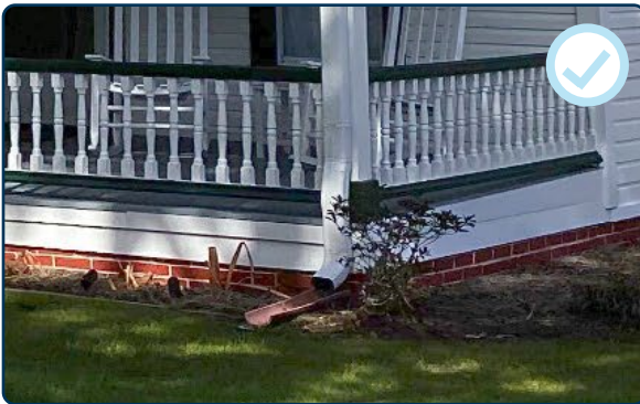
Figure 88: Appropriate downspout extension leading water away from building foundation.
