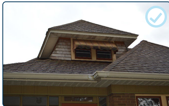
Figure 125: Appropriate awning over residential windows, this example just in need of basic maintenance.
