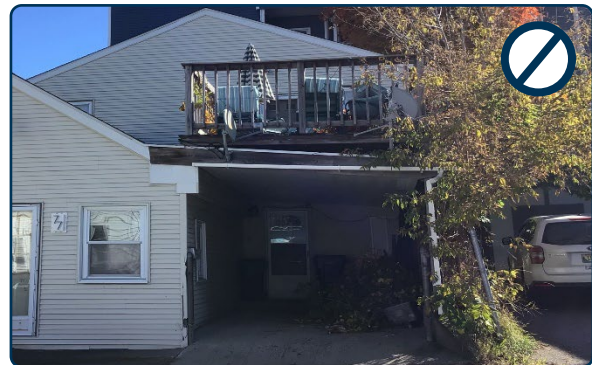
Figure 81: Inappropriate deck addition to the front façade of a residence.
