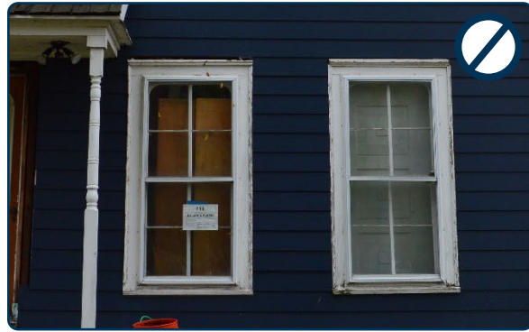
Figure 67: Inappropriate replacement windows that don't fit in the historic casing.
