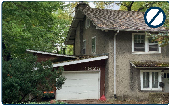
Figure 112: Inappropriate side addition with an incompatible roof shape.
