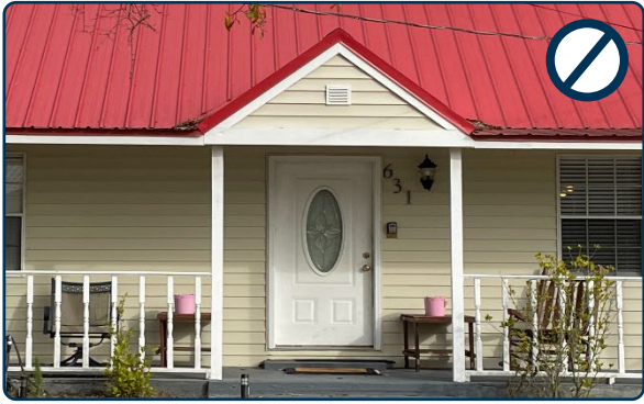
Figure 62: Inappropriate replacement of a historic door.
