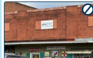
Figure 101: Inappropriate removal of contributing windows on the upper façade of a historic commercial building.
