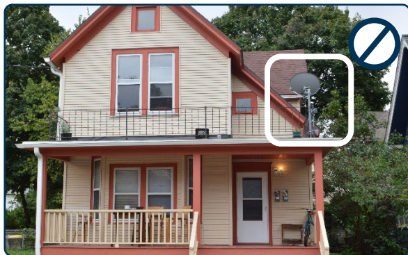
Figure 104: Inappropriate location of a satellite on the front façade of a historic residence.
