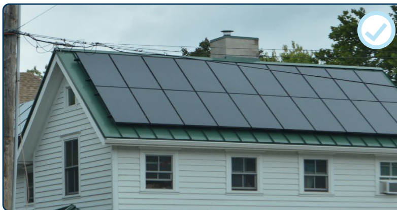
Figure 116: Solar panels installed on the metal gable roof of a residence.
