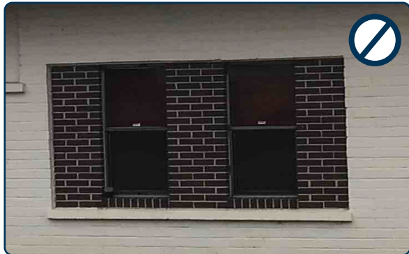
Figure 86: Inappropriate window infilled with masonry and new windows..
