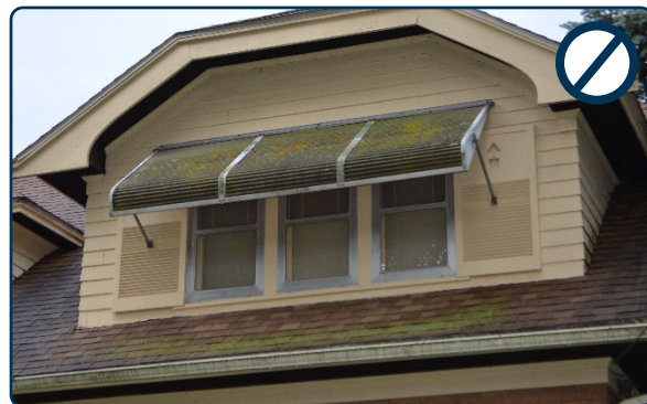
Figure 113: Inappropriate awning installed on top of window shutters.
