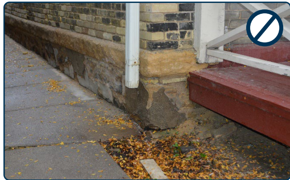
Figure 89: Improper drainage gutter system resulting in deterioration of foundation walls.
