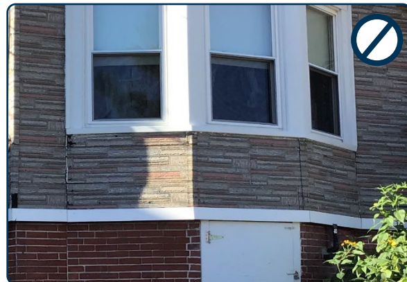
Figure 52: Incompatible rolled asphalt siding of historic residence.
