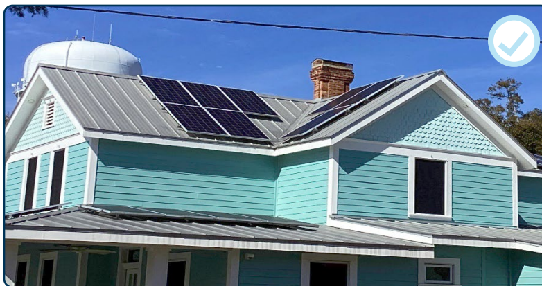
Figure 127: Solar panels installed on the metal roof of a residence.
