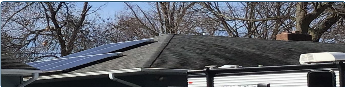
Figure 95: Example of solar panels appropriately installed on an asphalt shingle roof of a residence.
