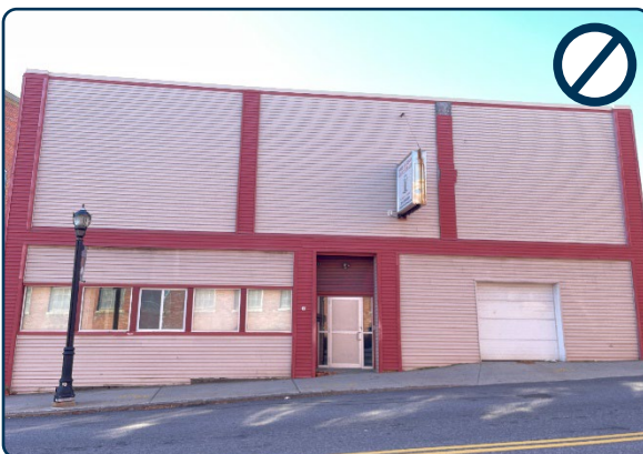
Figure 67: Example of inappropriate siding completely obscuring a historic commercial building.
