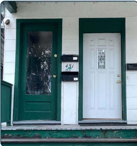
Figure 124: Inappropriate replacement door (right) that does not convey the architectural style of the residence.
