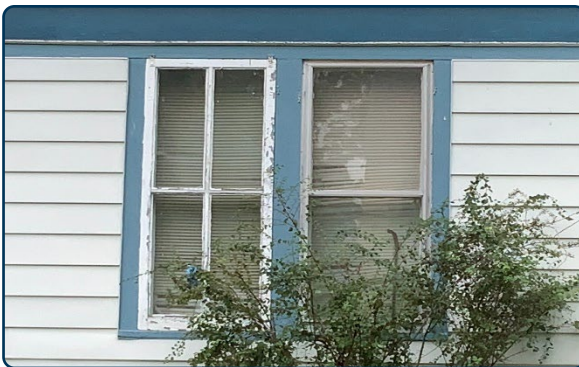
Figure 144: Inappropriate replacement window (right) that doesn't match the original.
