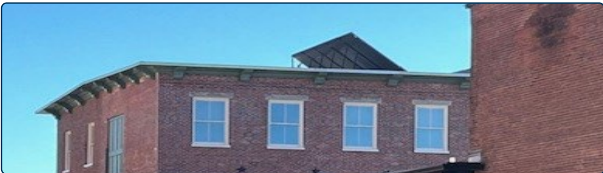
Figure 112: Example of solar panels installed on the roof of a historic commercial/industrial building
