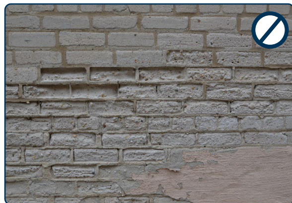
Figure 72: Inappropriate modern mortar replacement on a historic masonry building resulting in damaged bricks.
