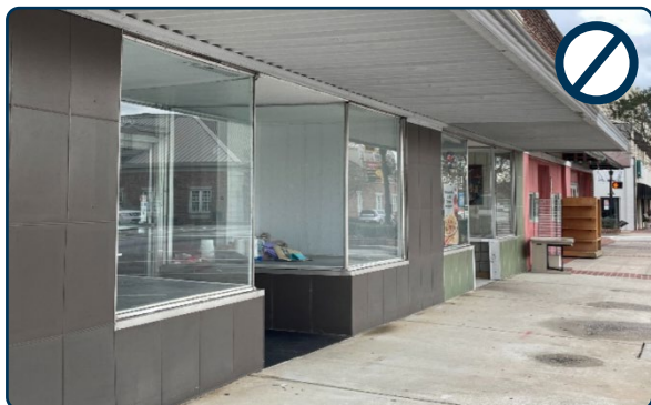
Figure 98: Historic storefront that has been inappropriately replaced.
