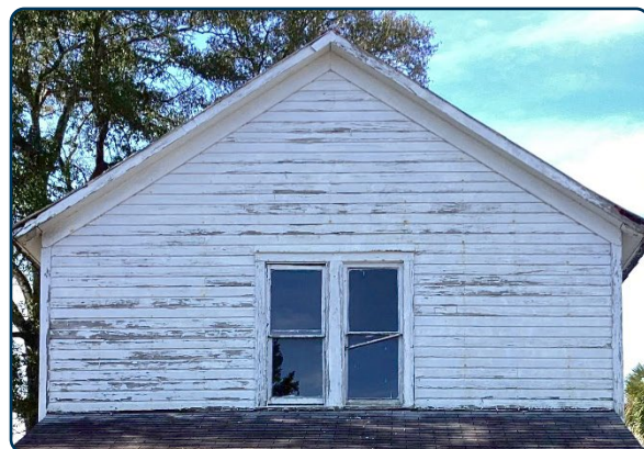
Figure 61: Example of wood siding needing to be re-painted and wooden windows in need of repair.
