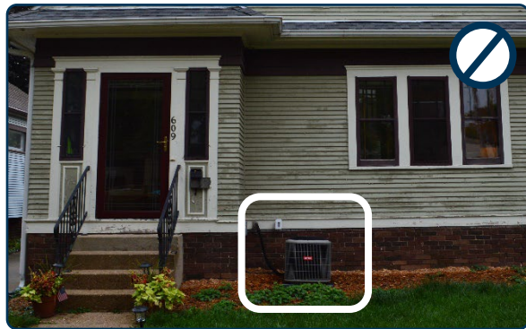
Figure 91: Inappropriate new air conditioner installed on the front façade of a residence that is not obscured behind screening or landscaping.
