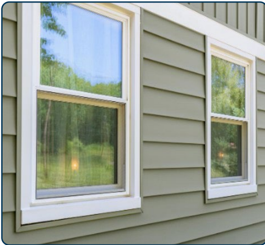
Figure 54: Example of more appropriate vinyl siding that uses smooth boards with compatible board length, width, and thickness.
