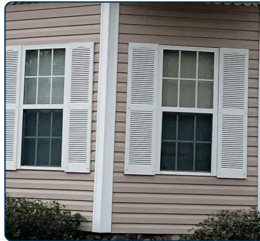
Figure 55: Example of inappropriate vinyl siding with incompatible board width.
